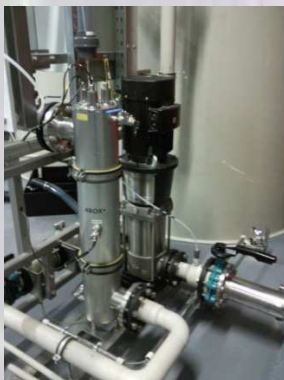
UV disinfection of process water
