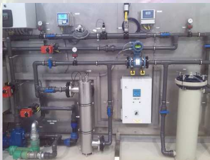
UV disinfection of process water
