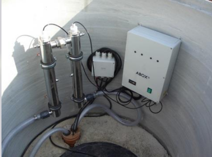
UV sterilisation of waste water
